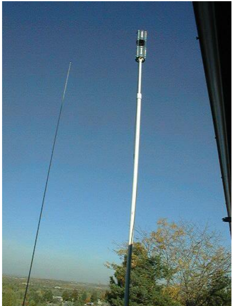
Antenna shown mounted on an 8 ft PVC pole on the Balcony Railing
